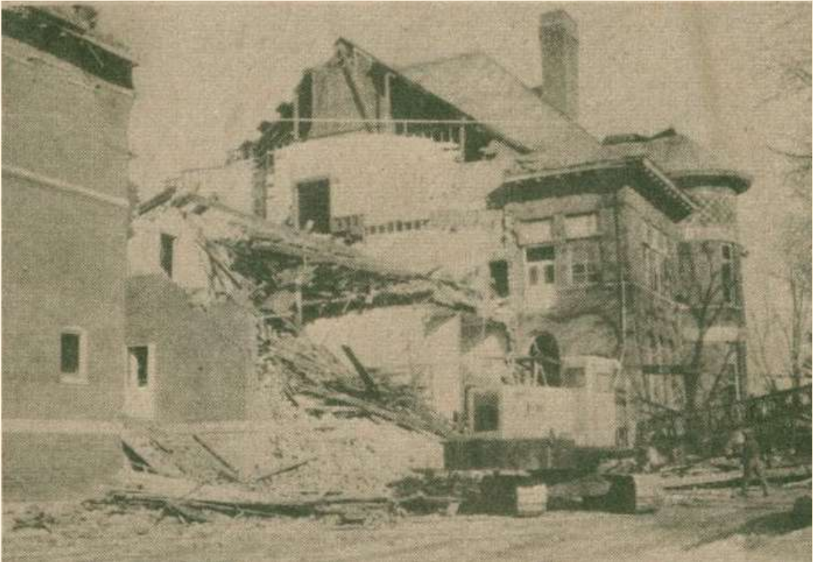
Old Engineering Building in Ada High School, 1953 – 1971 Demolition by Village of Ada
